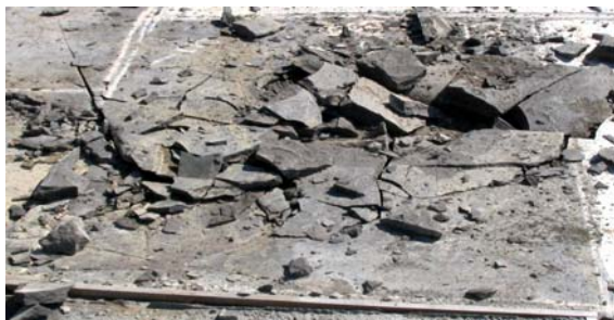
Unsupported rock surface
