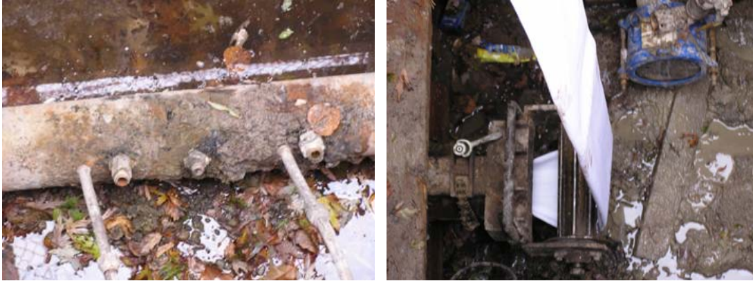
Corroded water pipe, Hamilton 2003. Liner repair, Hamilton 2003.
