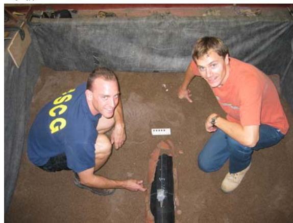
"MSc Student Brian Lapos (left) and Richard Brachman inspect a pulled-in-place polyethylene pipe (black) following an experiment. Pipe bursting was used to break away an existing clay pipe (red) to make way for the new polyethylene pipe. Ground displacements, pipe strains and pulling forces were monitored during the experiment."
